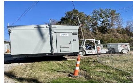
In St. Louis County, crews replaced Switchgear at a 50+ year old substation to support reliability for over 10,000 customers.
