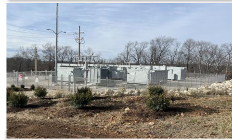
To meet the growing community's energy needs, a new substation, constructed in 2023, will benefit over 2,500 customers at the Lake of the Ozarks
