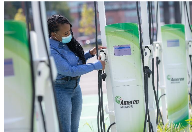
Charging stations at St. Louis Union Station placed in-service in 2020 as part of Ameren Missouri's Charge Ahead Program
