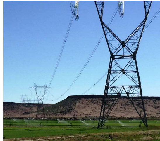
500-kilovolt (kV) transmission line near Melba, Idaho.
