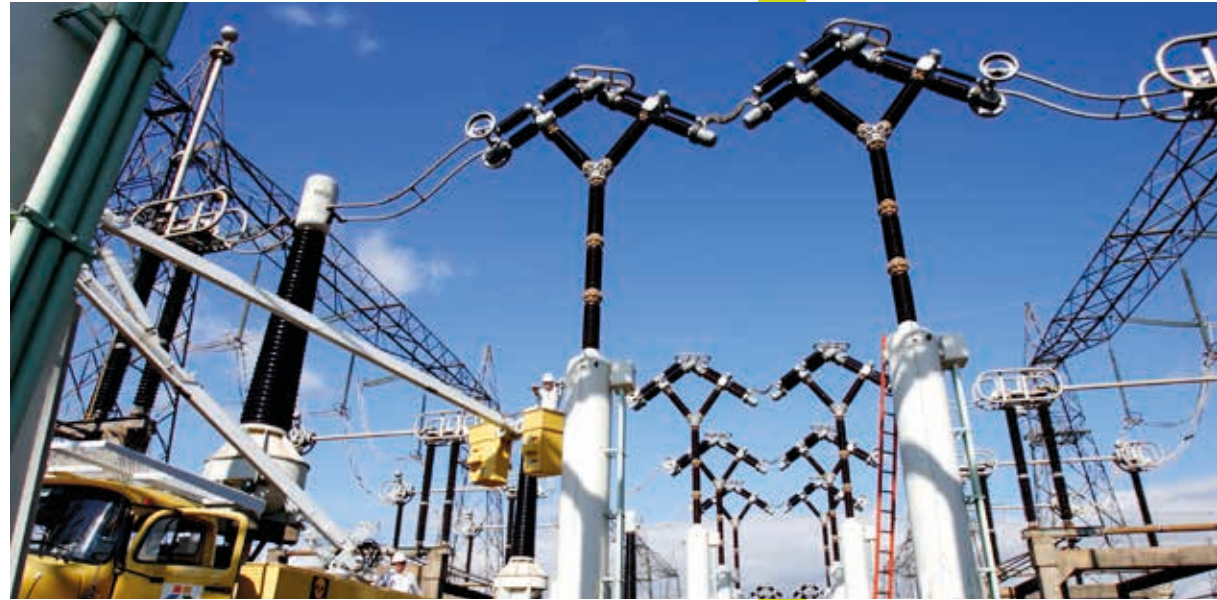
A substation at the Itaipu Dam. Photo by Caio Coronel
