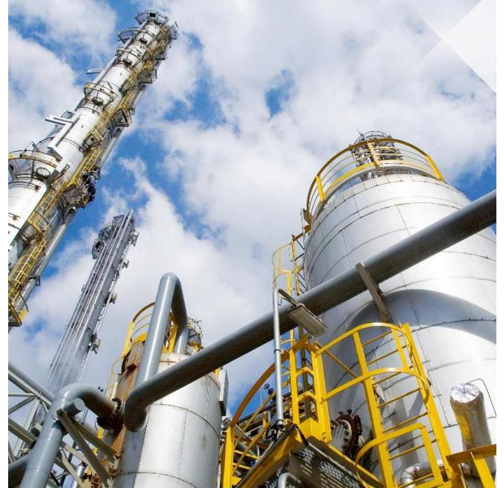
PKN ORLEN OLEFINS PLANT // PLOCK, POLAND
