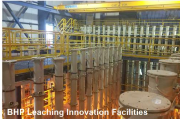
BHP Leaching Innovation Facilities 2024 Chilean copper site tour 18 November 2024
