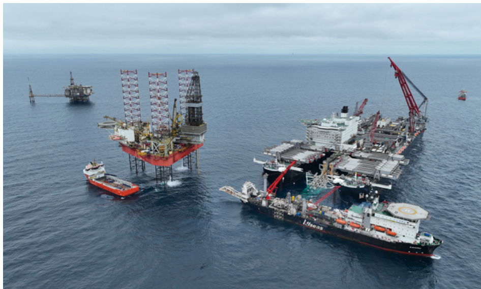
Installation of the Eldfisk North development at the Eldfisk Complex, part of the Greater Ekofisk Area.
