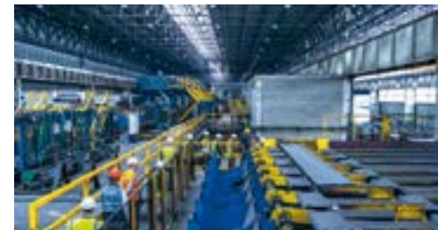
Acciaierie Venete / Italy The “Drawer” sizing-block for SBQ bars: perfect roundness and high operational flexibility.
