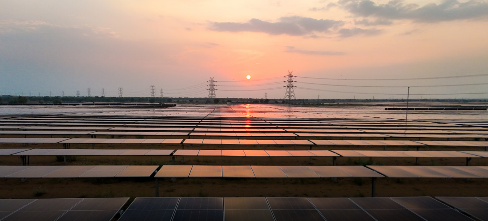
Nexttracker technology featured on Koppal Solar Power Plant, Karnataka, India
