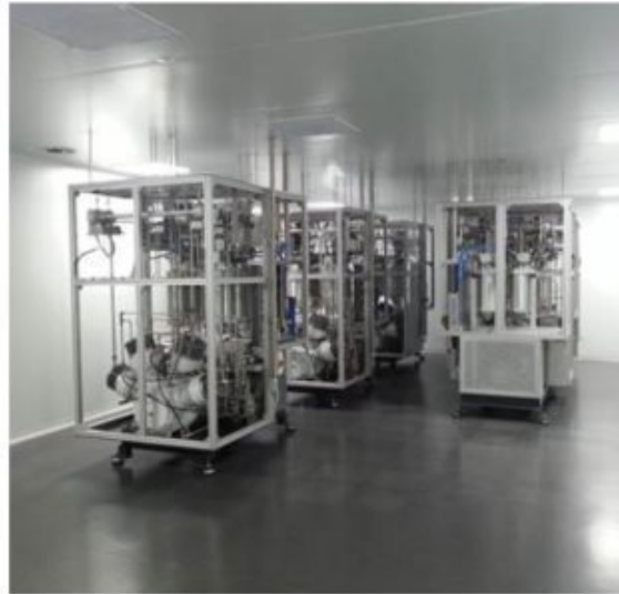
ASP's Carbon-14 enrichment facility
