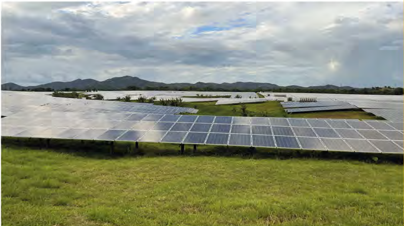
The Group's investment in the Monte Plata Solar Park in the Dominican Republic is part of our modern energy agenda
