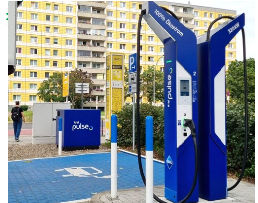
Berlin: Installed at a Gas station downtown
