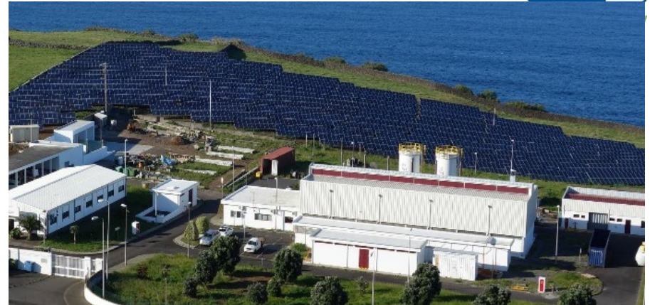
Isolated Off-Grid Power Plant; managing very large-scale mixed feed while Battery Buffering System provides multi MWhrs of capacity.
