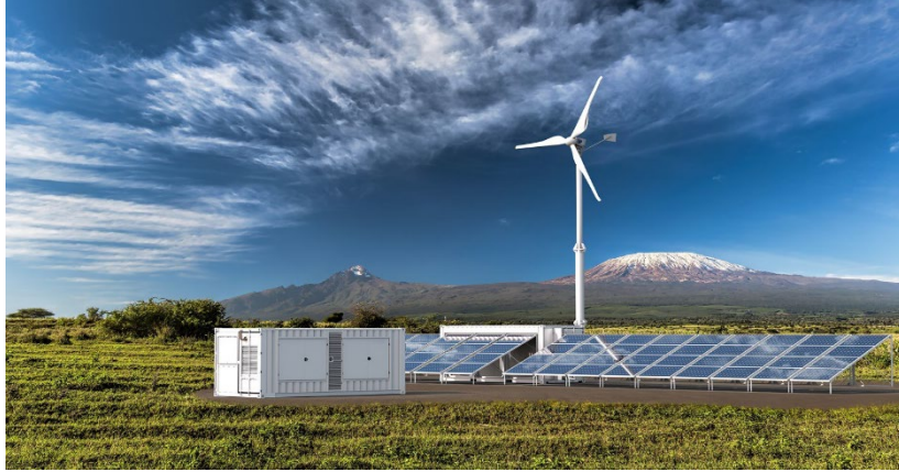
Microgrid in Lithuania; managing mixed input feed while Battery-Buffering System provides 150KWhr.
