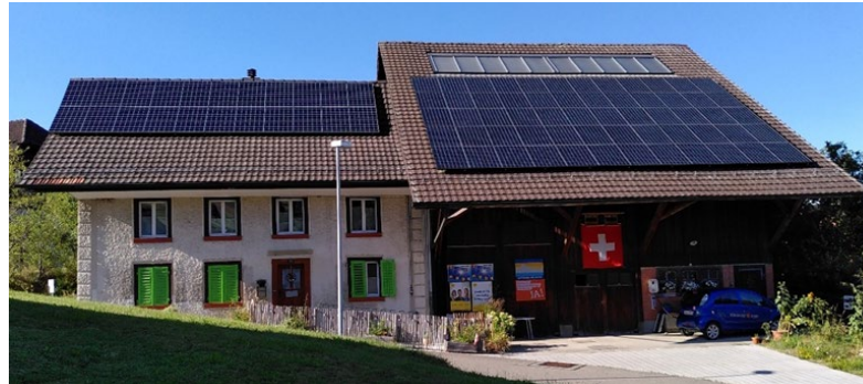
Home Power Plant in Switzerland; Battery Buffered System providing 9MWh (year 1): PV, Solar, Thermal, Storage
