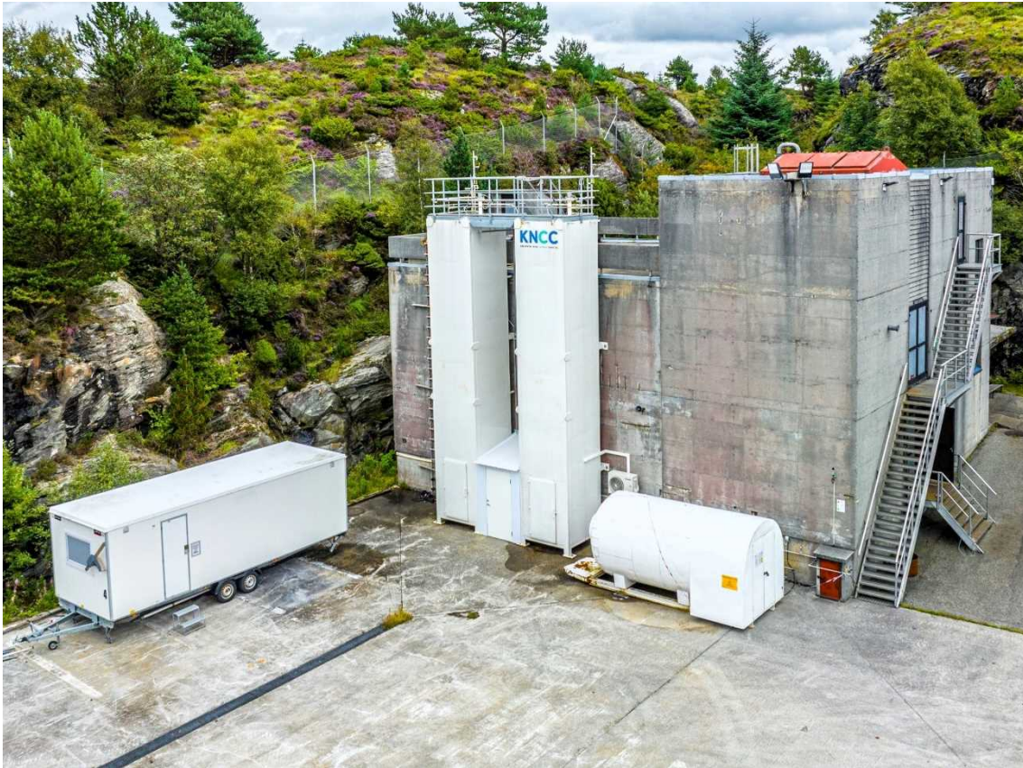
KNCC's demonstration facility (CTC test rig)
