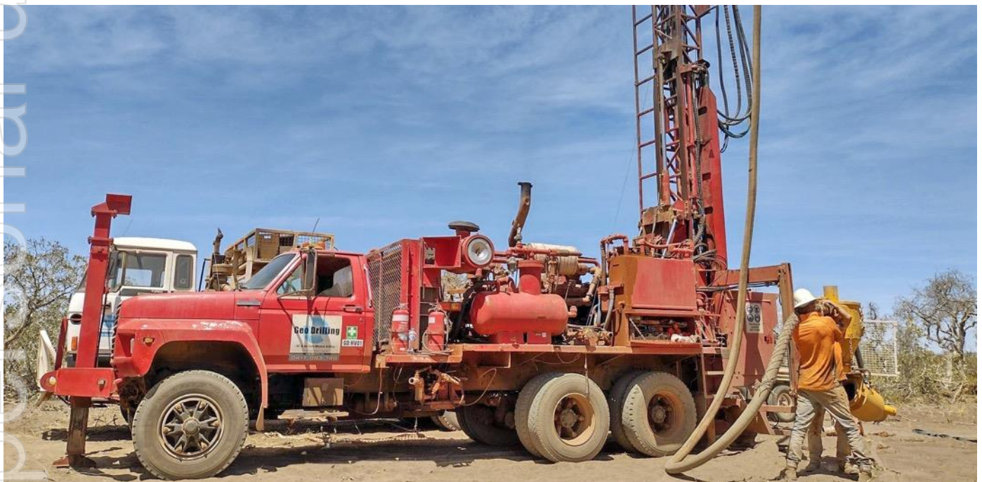
Figure 1 Drilling rig setting up on the first drill collar of the Benmara Project September 2021
