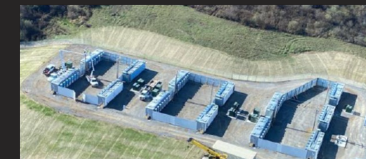
B HOPEDALE, OH 22MW ENERGIZED CAPACITY
