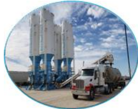
Wellsite Storage Solutions
