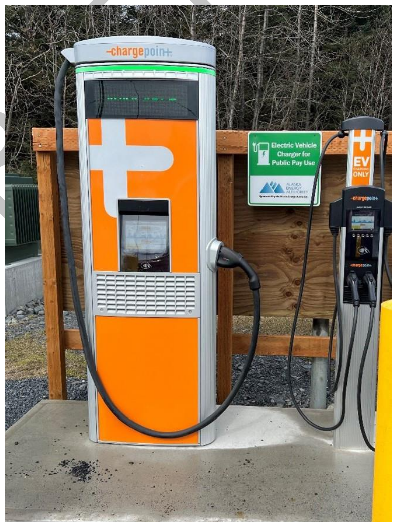
AEA-funded EV charging stations in Seward Photo courtesy of AEA
