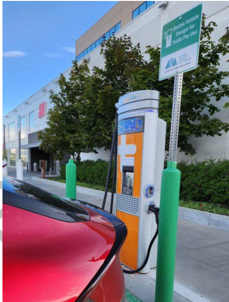
Charging station at the Dimond Center, Anchorage Photo courtesy of AEA
