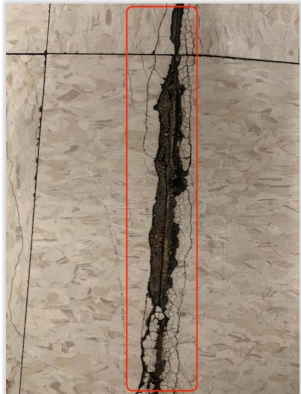
Photo 4. Clinic floor damaged and unsanitary (photographed on 4-10-23).
