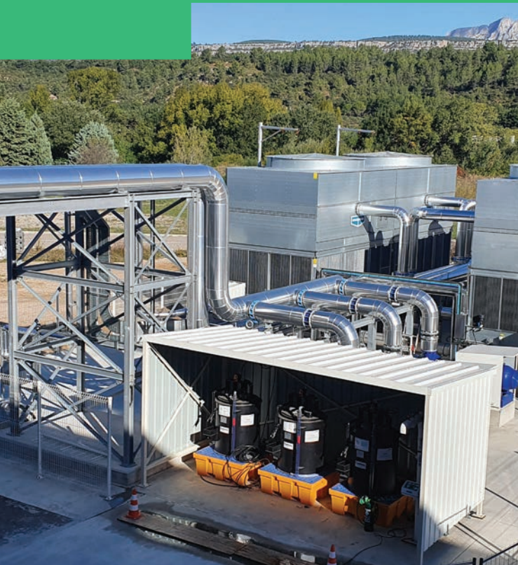
Aerofree cooling equipment, ST Rousset, France
