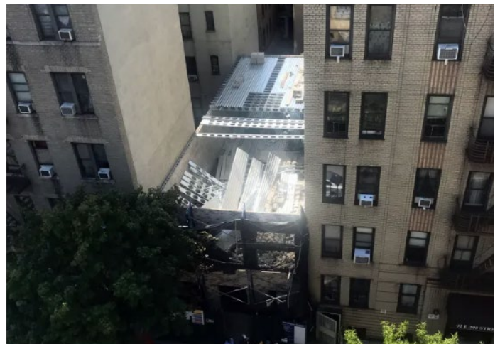
A VIEW OF the collapse that happened at 94 E. 208th St. in Norwood where one worker at the building died. Photo by David Cruz
