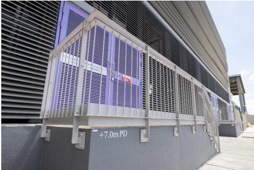
The floor of the gas-fired generating unit L12 has its foundation built to a +7.0 metres PD specification, significantly reducing the risk of flooding.
