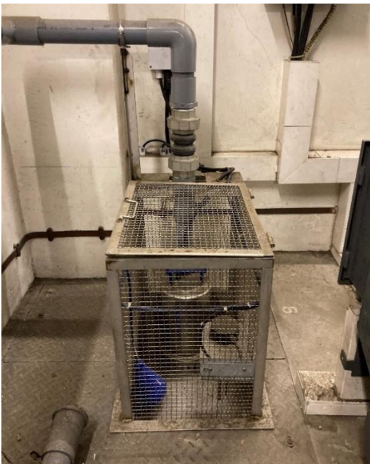
Automatic water pumps and flood alarm systems are installed at existing distribution substations.
