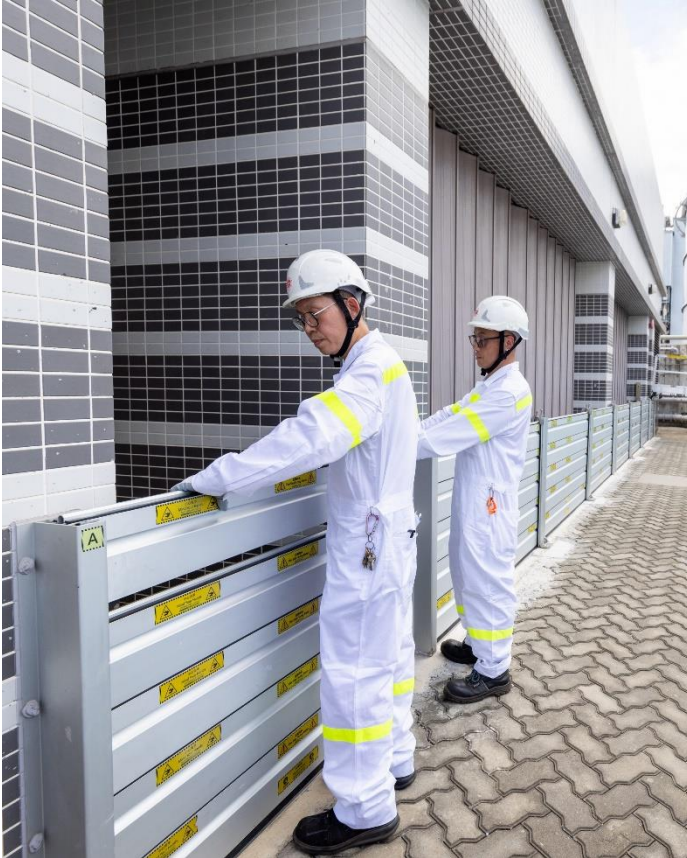
Demountable floodgates are being used to protect critical power generating facilities and auxiliary installations.
