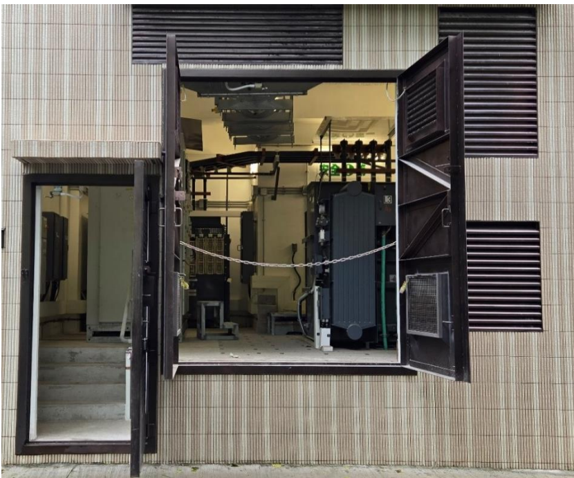
The floor level of all new substations is raised to enhance flood protection.
