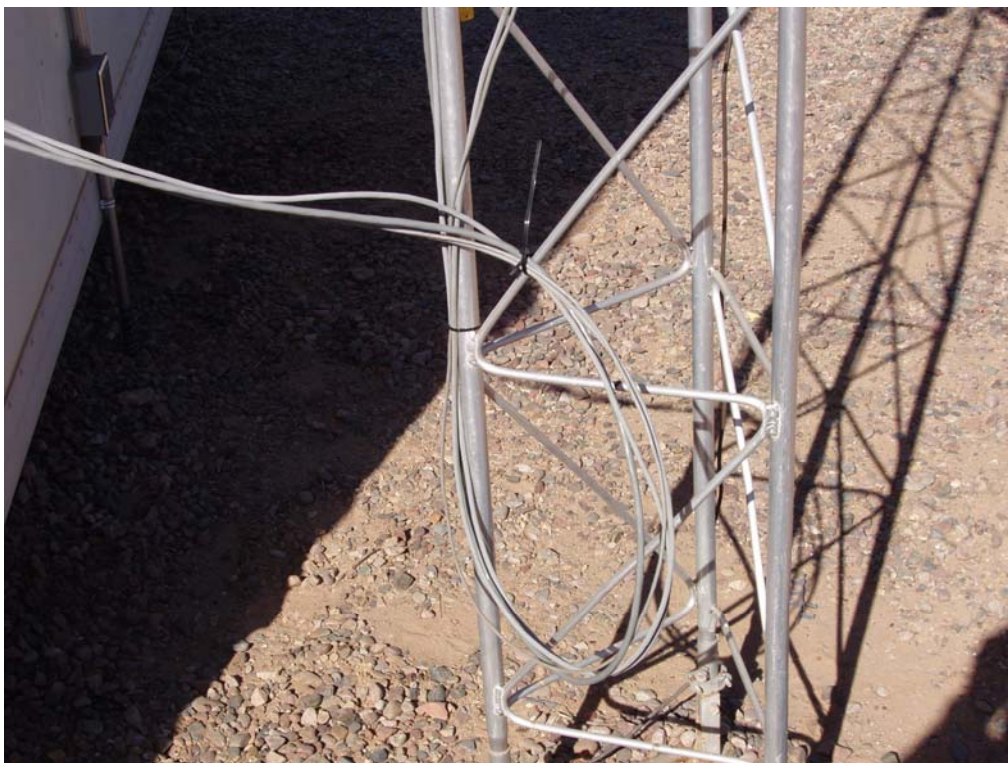
Figure 1.13 Signal Cable at Tower Base
