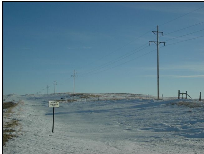
Figure 2-14 Existing Verendrye Power Line at Highway 23 Crossing
