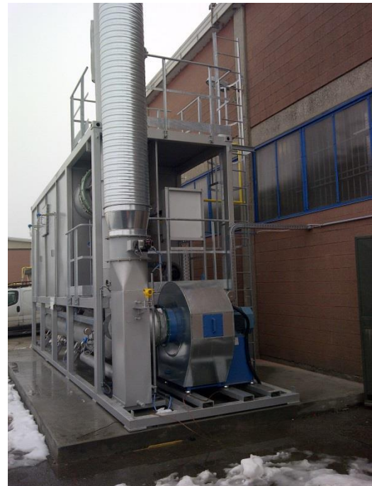
RTO10 recently installed by Donau Carbon in Italy
