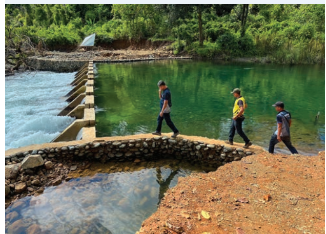
USAID Philippines supported the Palawan government to develop a climate-resilient water intake structure to supply water. Credit: USAID
