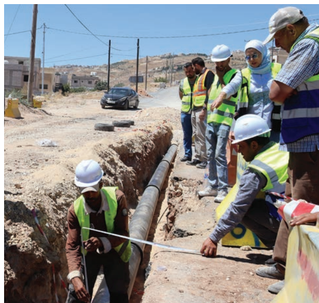
USAID Jordan improved the country's water supply network by replacing outdated components and installing smart meters and leak detection equipment. Credit: USAID
