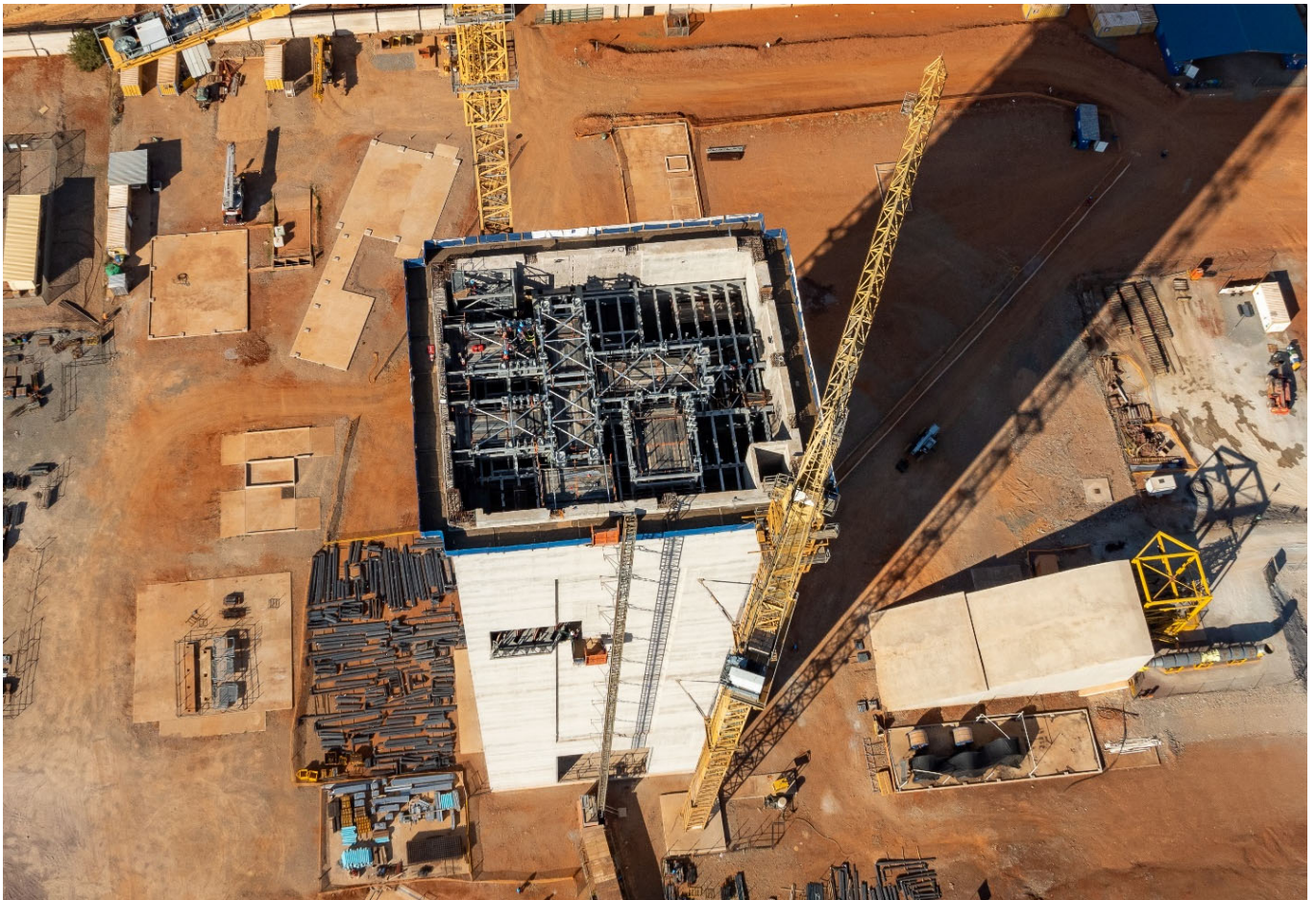
Photo: Structural steel erection in progress at Shaft 2. The 10-metre diameter Shaft 2, which is required for the Phase 2 expansion, will be the largest hoisting shaft on the African continent.
