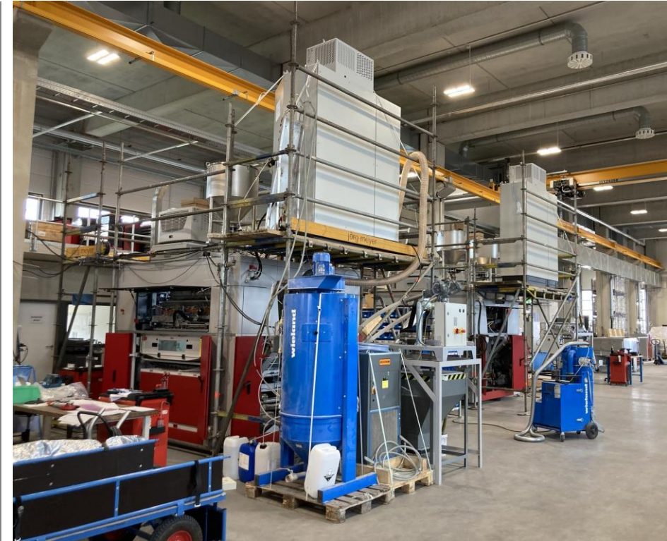
Picture taken in VJET headquarters in Germany, April 2021: assembly of VJET X units 4 and 5
