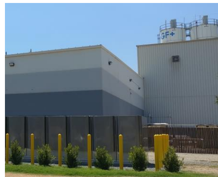
Bloom Energy Servers deployed at a California manufacturer
