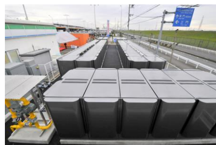
Bloom Energy Servers deployed at the Osaka Fish Market in Japan
