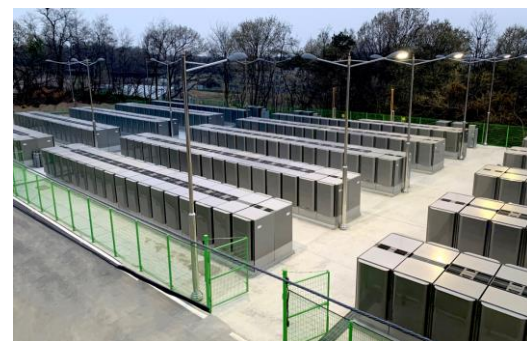
19.8 megawatts of utility-scale Bloom Energy Servers in Hwasung, South Korea.
