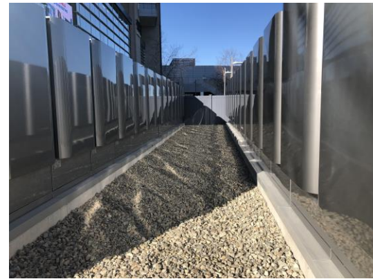
2 megawatts of Bloom Energy Servers at Gillette Stadium, Foxborough, MA.
