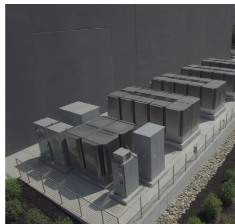
Bloom Energy at a data center
