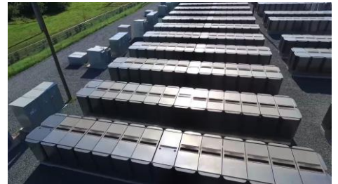
Bloom Energy Servers deployed at utility scale
