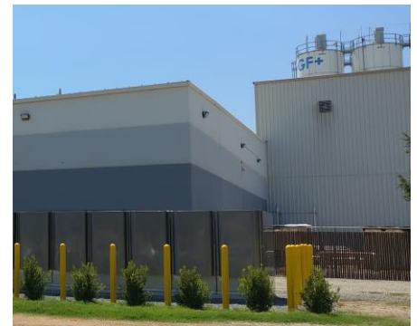
Bloom Energy Servers deployed at a California manufacturer
