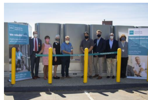
Ribbon cutting for newly installed Energy Servers at Hospital for Special Care in New Britain, CT.
