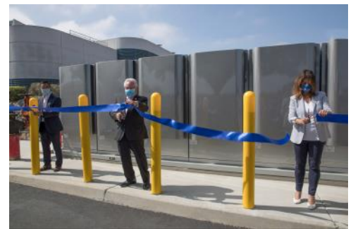
Two AlwaysON Microgrids were powered-on for SoCalGas facilities in the Los Angeles-area, followed by a ribbon cutting. Pictured, left to right: Kris Kim, Bloom Energy; California State Senator Bob Archuleta; Maryam Brown, SoCalGas. Photo credit: SoCalGas/Lance DeLaura
