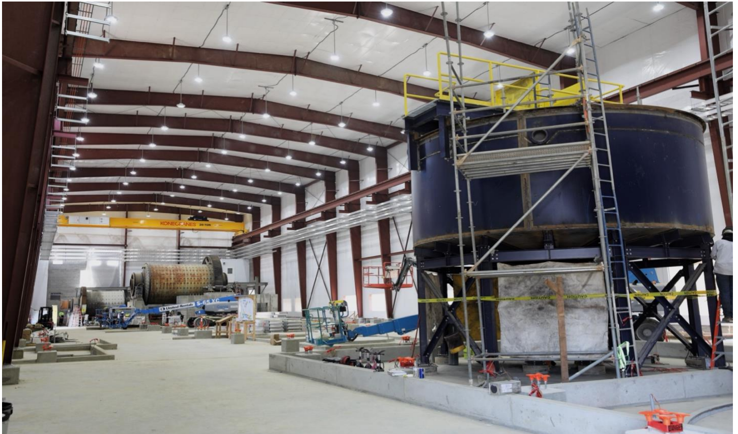
Figure 1 - Interior of mill facility with lead concentrate thickener in the forefront and ball mills in the background
