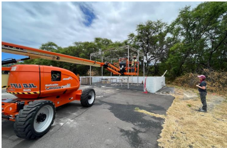
Figure 3-1. Passive acoustic bat detector being installed under supervision of Sandia bat biologist
