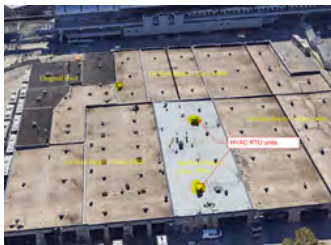
Aerial view of the Frankford Depot roof which needs replacing.
