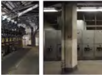
Images of the current Market St. Substation.
