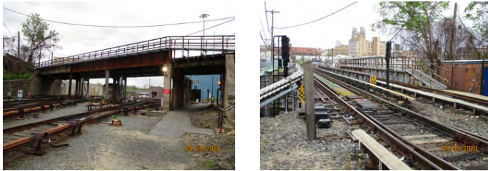
Image of the Norristown High Speed Line Bridge 0.15 over the 69th Street Yard Tracks.
