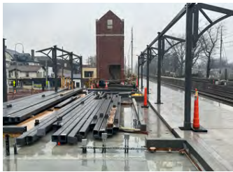
Construction at Ardmore Transportation Center on the future elevator wall and canopy.
