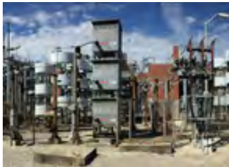
Image of the current static frequency converters at Wayne Junction, all of which are near the end of their useful life.
