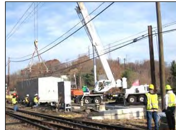
Signal Hut at River Interlocking Manayunk/Norristown Regional Rail Line
