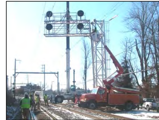
Signal System Modernization Warminster Line
