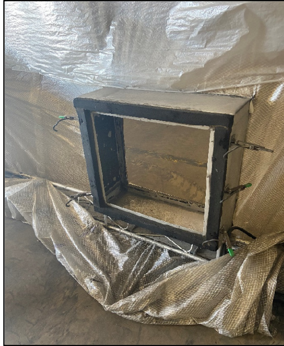
Photograph 3: Exhaust connection point on lowered shroud, Warehouse F.
