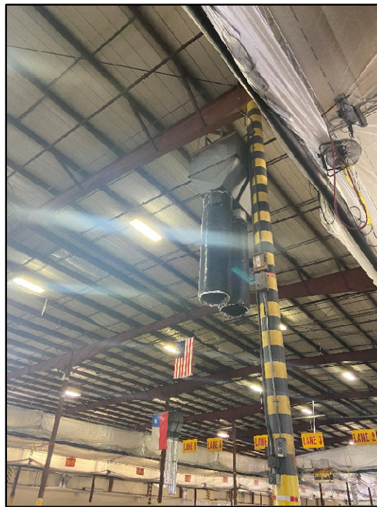
Photograph 6: Exhaust blower, shroud fan and flexible hose connections, Warehouse F.
