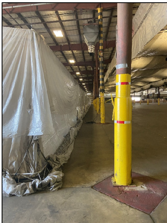
Photograph 8: Lowered shroud and blower connection point without flexible hoses.
