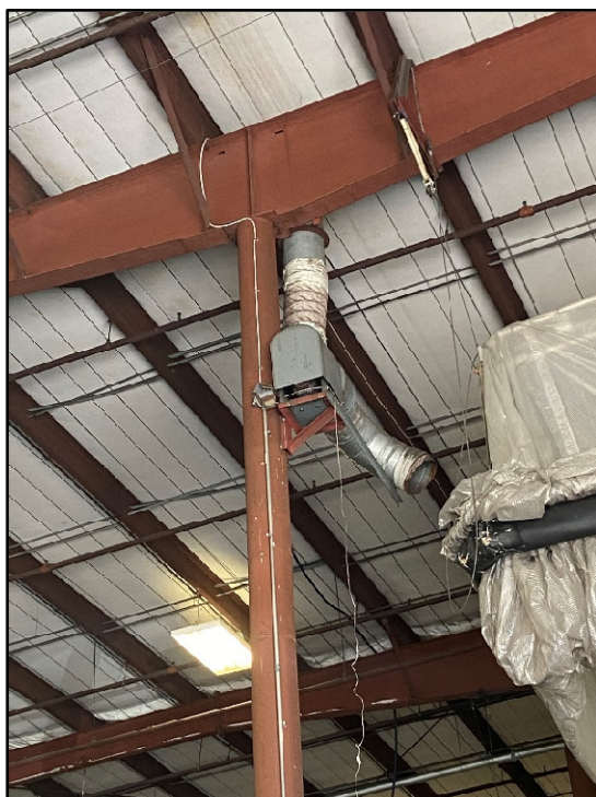
Photograph 9: Blower and connection point without flexible hose, Warehouse F.
