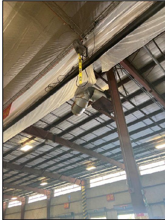
Photograph 5: Exhaust blower and shroud fan in elevated shroud, Warehouse F.
