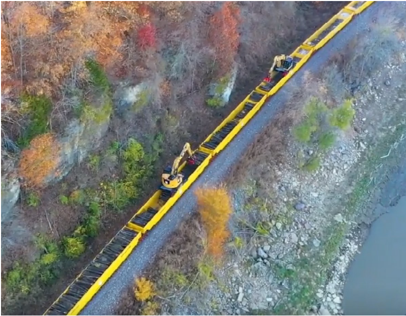
We are speeding up our used rail tie pickup process with specially designed work equipment to enhance safety and efficiency. We annually divert 90% of our used railroad ties away from landfills to energy recovery facilities.
