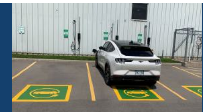
Electric vehicle charging stations at the Mold-Masters Georgetown location.
